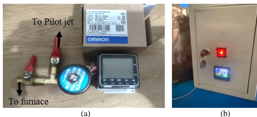
Figure 3. (a) Selenoid Digital Temperature, (b) Panel Box Control
