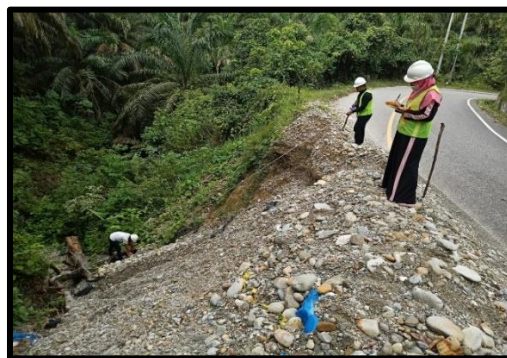
Figure 1. Landslide Location on Subulussalam-Lipat Kajang Road
