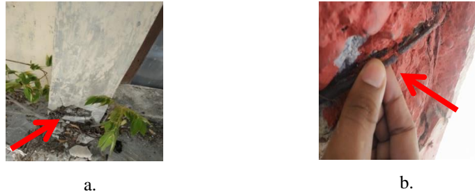
Figure 3. a. Spalling on Columns, b. Broken stirrup
