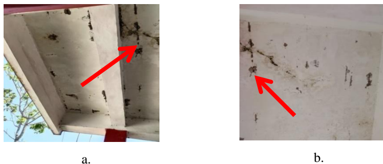
Figure 5. a-b. Spalling On Plate
